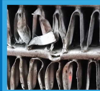
8. Close-up of damage site
