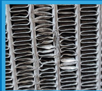
7. Place of leakage
